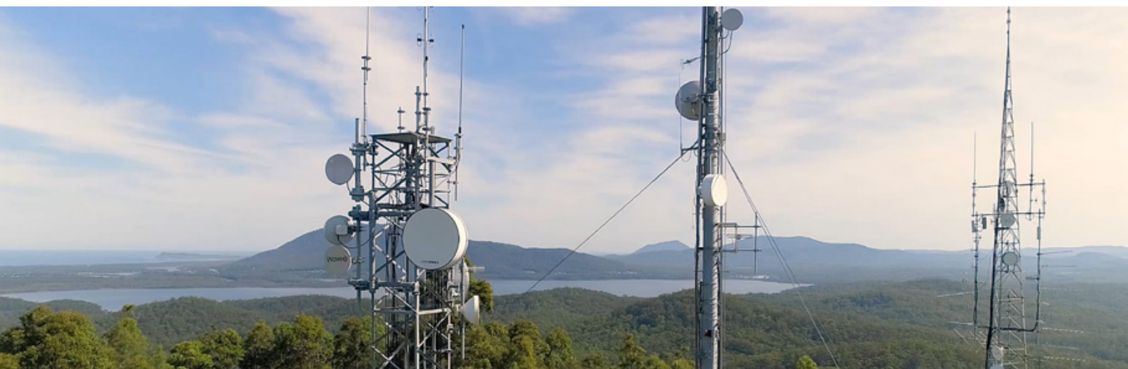
Critical Communications Enhancement Program, NSW Telco Authority
